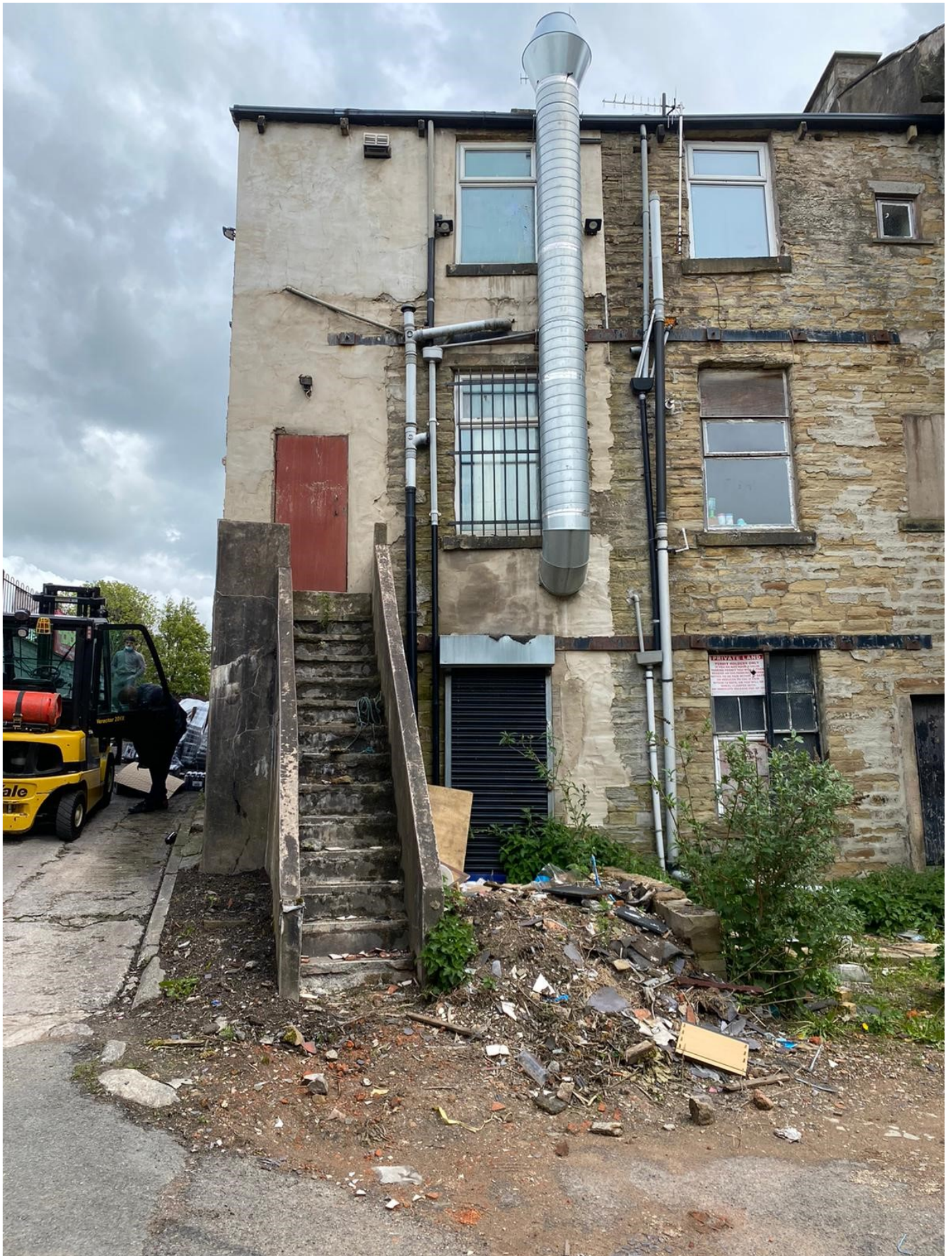
Dropped a pallet on public path and on my gable wall on 24th May 2021
